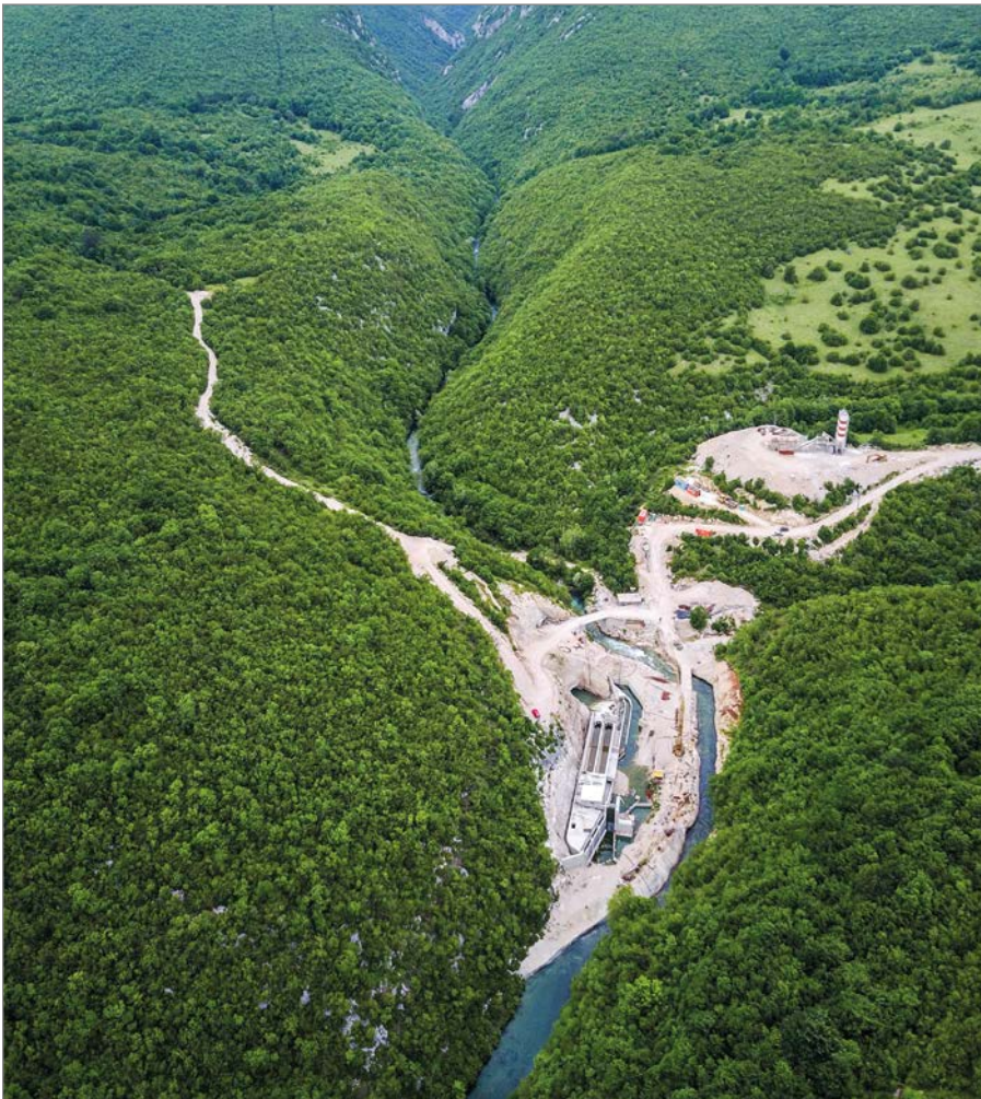
Construction of the Medna Sana hydropower plant near the source of the river Sana, Bosnia-Herzegovina. The Sana is one of six most important rivers for the huchen, a globally endangered fish species (photo by Matic Oblac).
