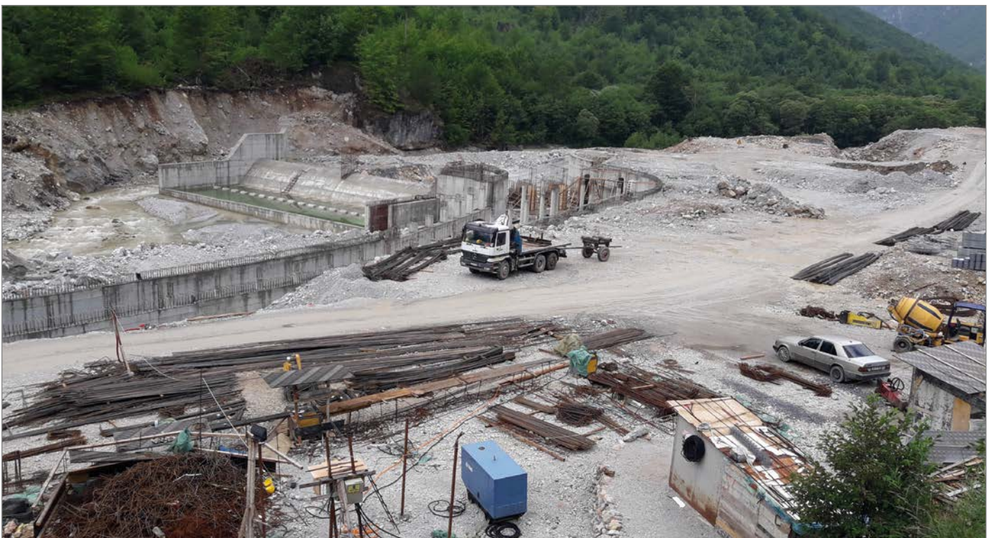
Dam construction site at the Valbona, in northern Albania. Construction continues even though the appeal court has ordered a construction freeze (photo by Cathrine Bohne).
